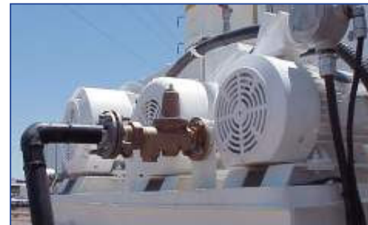
NOx Water Supply (2" pipe)
