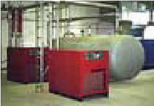
Air compressor station
