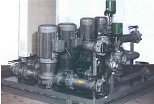
Water supply Module
